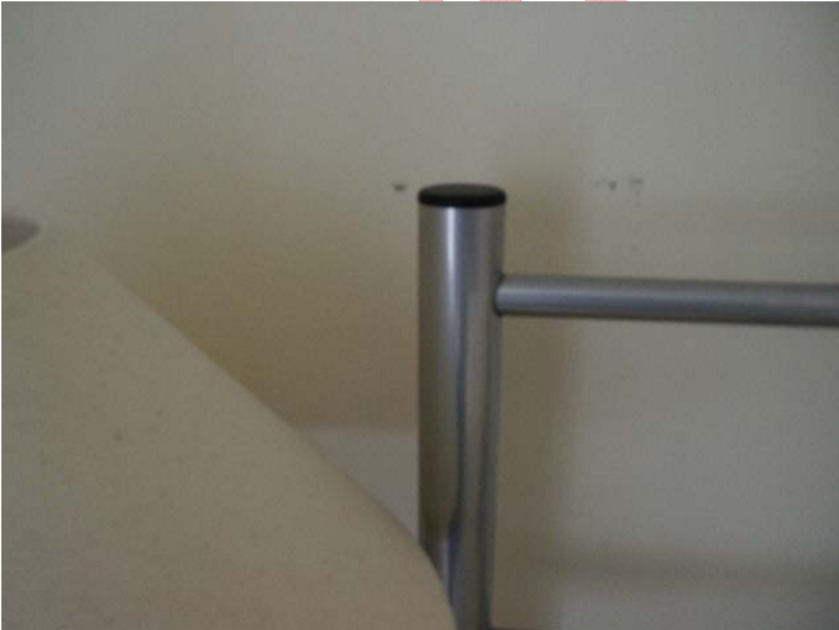
Bedroom – marks to wall behind headboard
